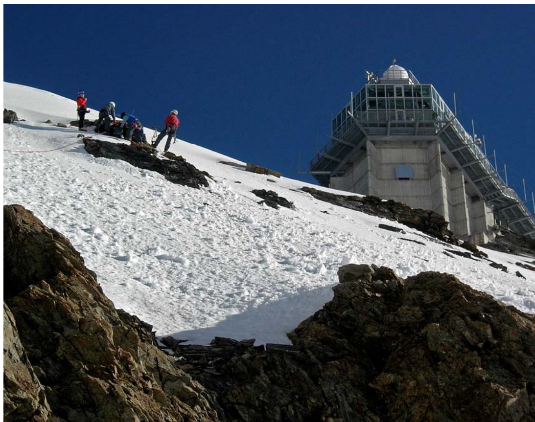
Photo 2: Installation of a sensor node between the roof of the research station and the Sphinx Terrace. This node is part of a PermaSense wireless sensor network prototype (photo: Andreas Hasler).
