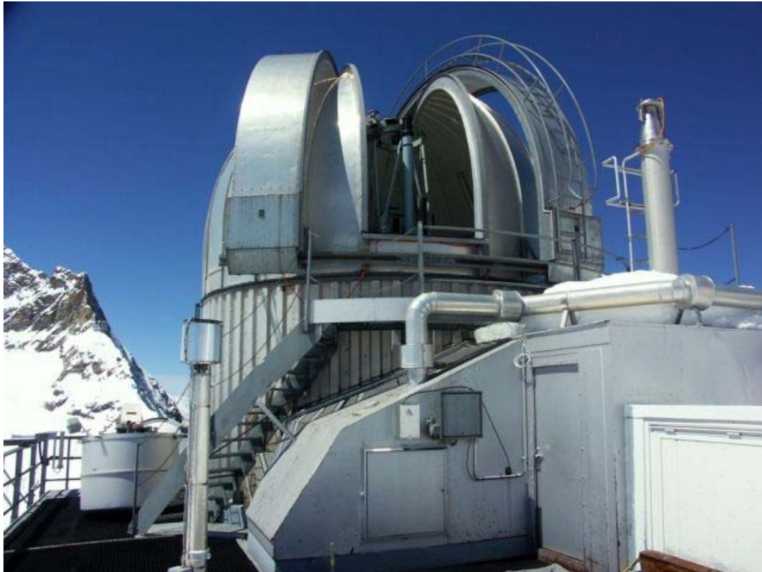
May: New use of the astronomical telescope in the Sphinx cupola at Jungfrauoch with EPFL's ozone differential absorption lidar (DIAL) receiver, under a clear sky.
