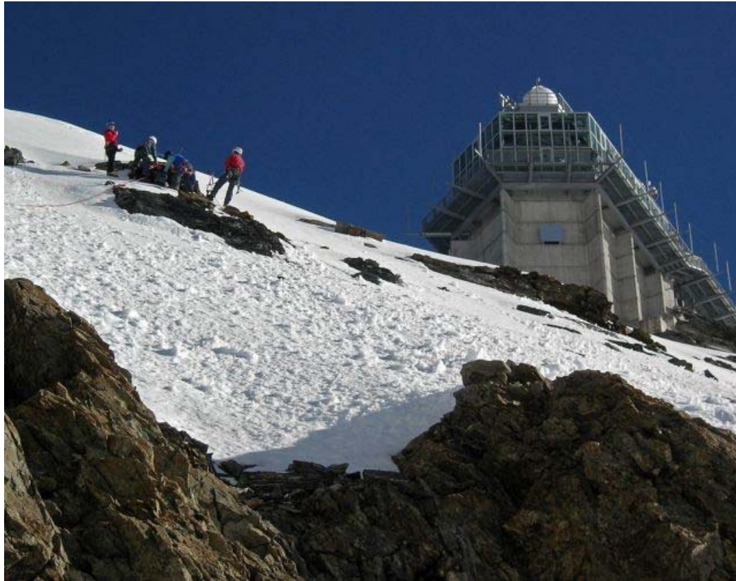
March: Installation of a sensor node between the roof of the research station and the Sphinx Terrace. This node is part of a PermaSense wireless sensor network prototype (photo: Andreas Hasler).
