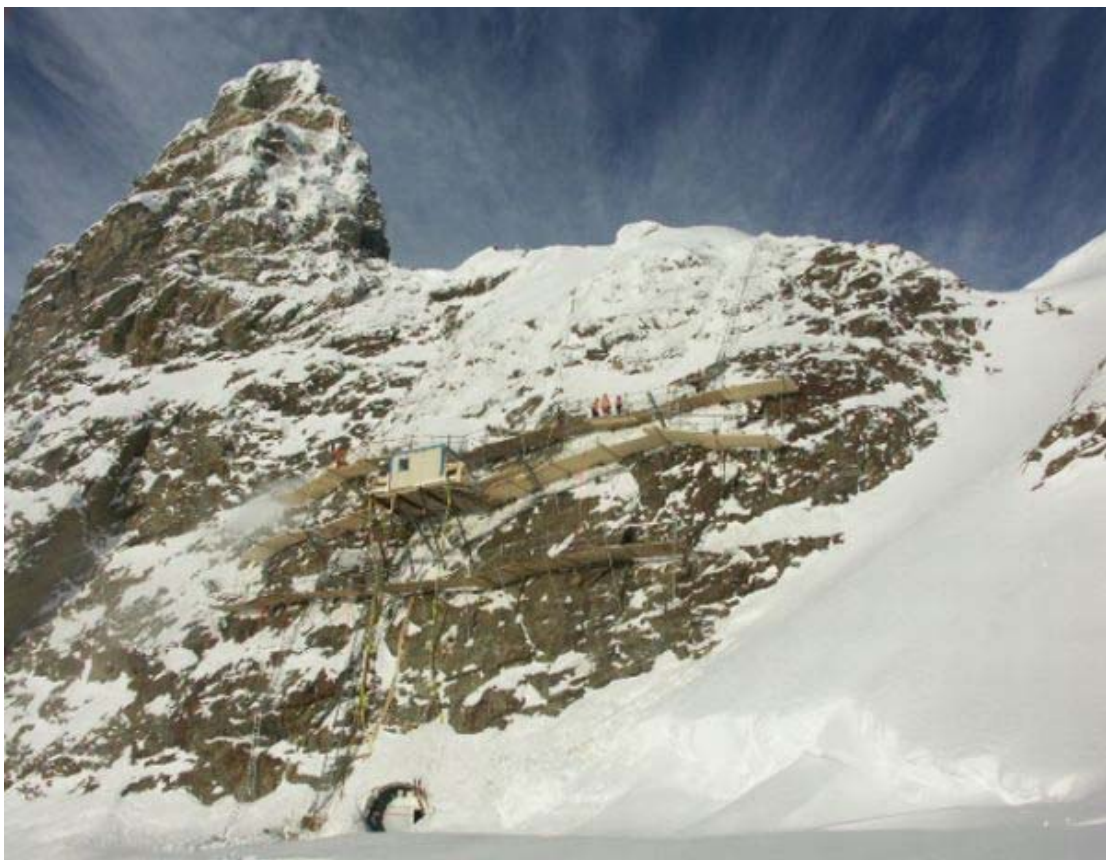
December: The Jungfraubahn's impressive efforts to secure the Sphinx rock above the Aletsch exit.
