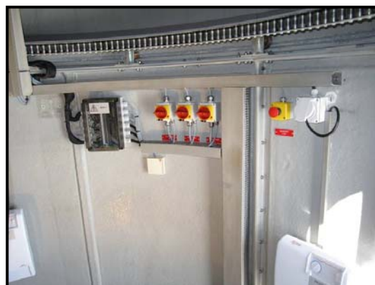
Figure 3: Safety switches for interrupting the motors
