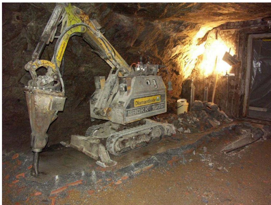
December: Reconstruction work in lab 10 at the research station Jungfrauoch during November and December.
