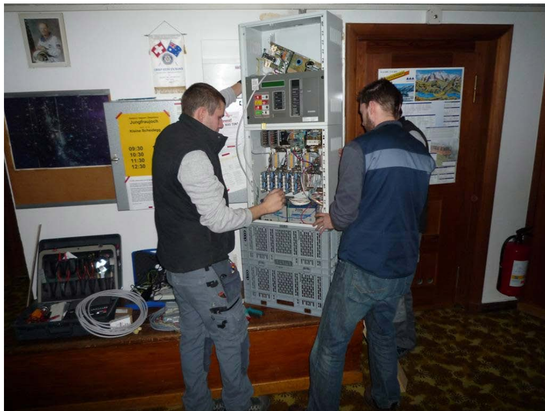
February: A new fire alarm system is being installed at the entire Jungfrauoch site. Here the installation in the Research Station by technicians from Aeschmann and Siemens.
