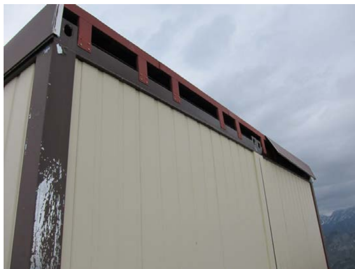
Figure 1: Defective roof of SONTEL lab container.
