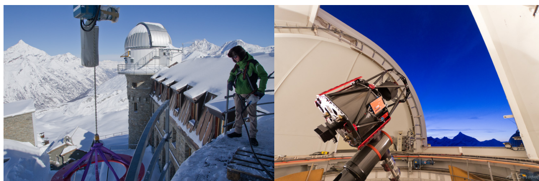
Figure 10. Installation of the base for the telescope mount on February 26, 2013 (left) and installation of the telescopes on June 6, 2013 (right) by the crew of the University of Bern at Gornergrat South observatory.
