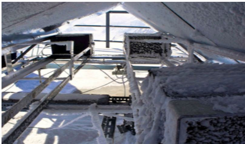
Figure 1. Prototype detector installed on the Sphinx terrace to test upward/downward particles' separation and environmental effects.
